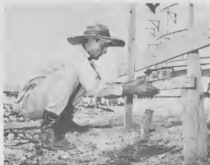
CONSTRUCTION WORK on Lago's new bunker station in Oranjestad nears completion. This lad is setting the level for a fire wall. TRABAHO DI construcion na e stacion nobo di bunker di Lago na Oranjestad ta haci bon progreso. E hoben aki ta aplica e waterpas na un muraya.
